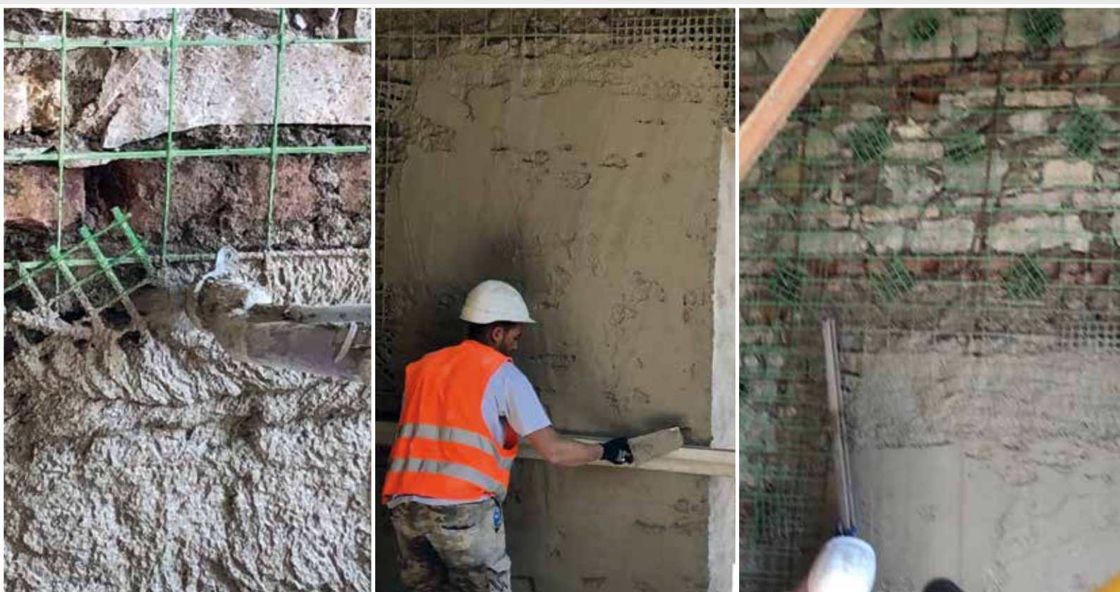
The reinforcement is completed through a layer of plaster based on NHL hydraulic lime
