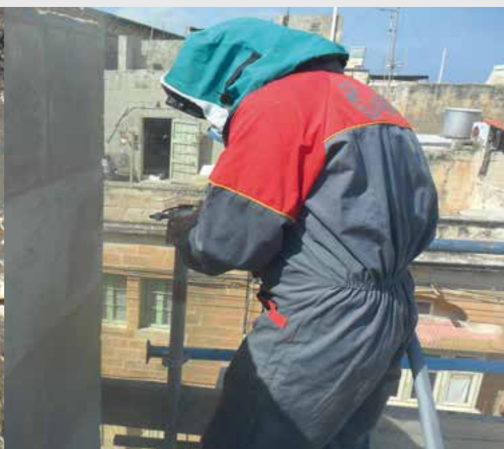
Restoration, removal of black crusts and salt efflorescences with HELIX® air-abrasion technology
