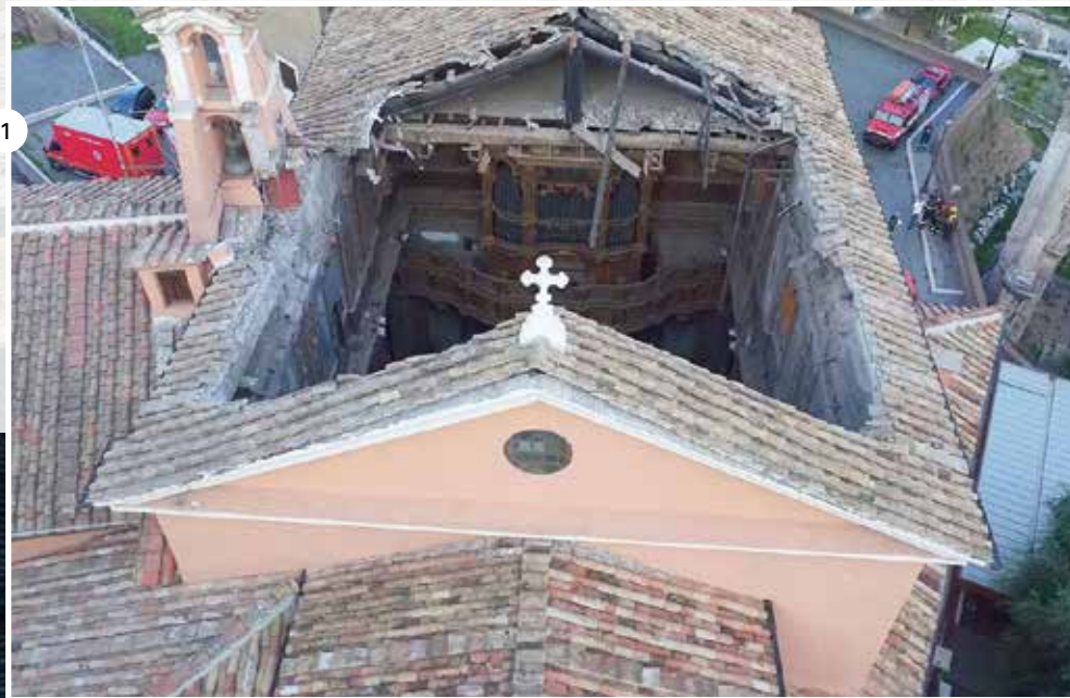
Fig 01. The collapse of the roof in a photograph of August 30 th , 2018, taken by the local Fire Department
