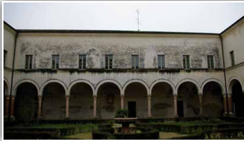
The northern façade of the Cloister of Secolari before and after the restoration
