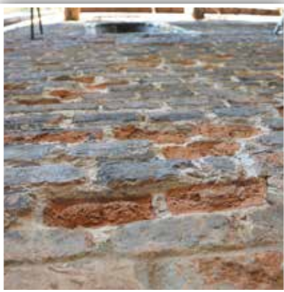
Figure 2. Juliet's house, decay of brick facade
