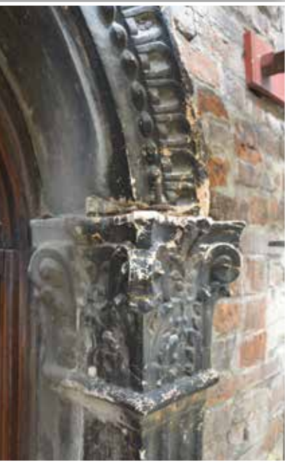
Figure 4. Juliet's house, particular of the decay of the stone frame: black crust
