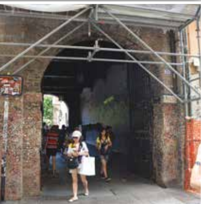
Figure 5 Juliet's house, particular of the entrance arch to the courtyard before restoration
