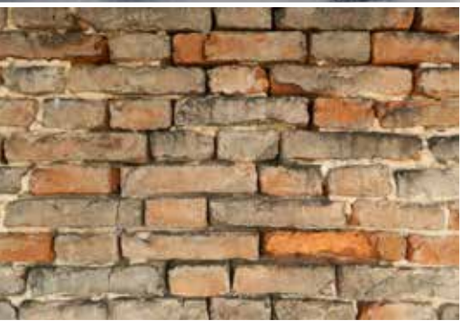
Leaching process of mortar joints, N-W facade
