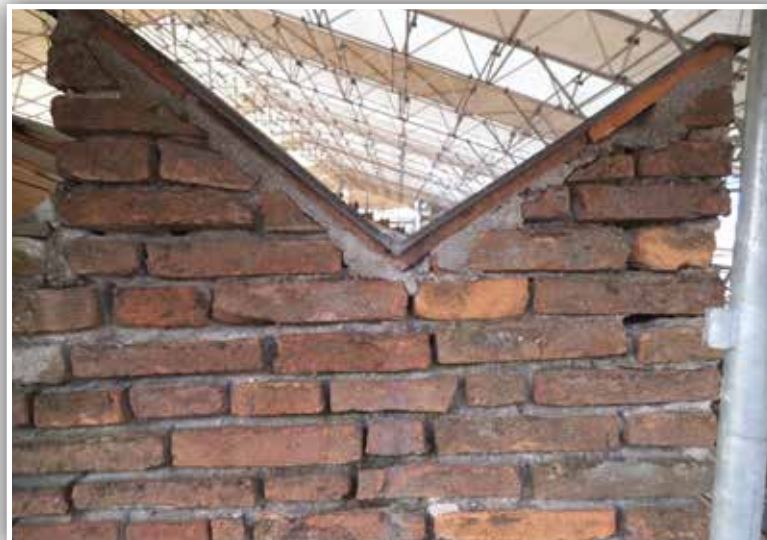
Degradation of merlons mortar
