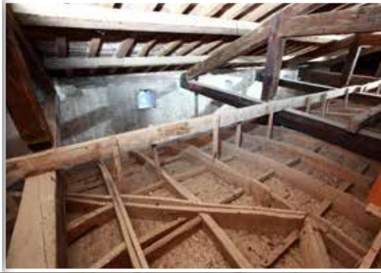
general view of the ceiling of the library and of the structure of the roof before the interventions
