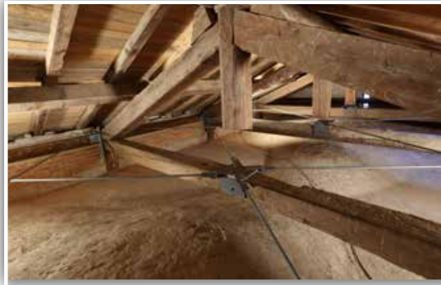
General image of the strengthening interventions on the roof over the "Scriptorium"
