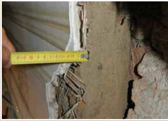
detail of a portion of ceiling collapsed during the earthquake.
