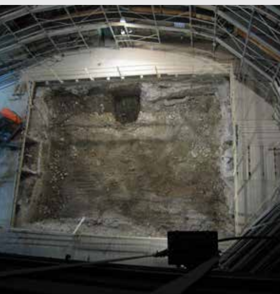
The excavation necessary to realize the water tank under the floor of the main hall.
