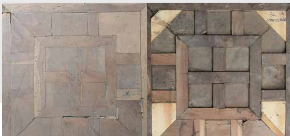
One of the tiles from Sala Quattro Stagioni before restoration, view of the front and back. Are obvious damage caused by wood-boring and old speeches of “restoration”
