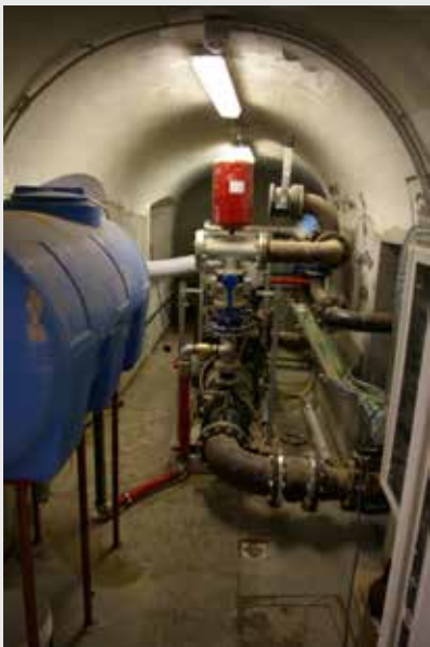
The room in the basement that hosts the main pump of the water sprinkler system
