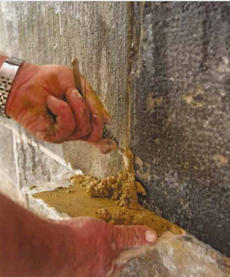
After careful analysis MAPE-ANTIQUE LC, cement-free, hydraulic binder based on lime and Eco-Pozzolan was used to repair the sandstone blocks
