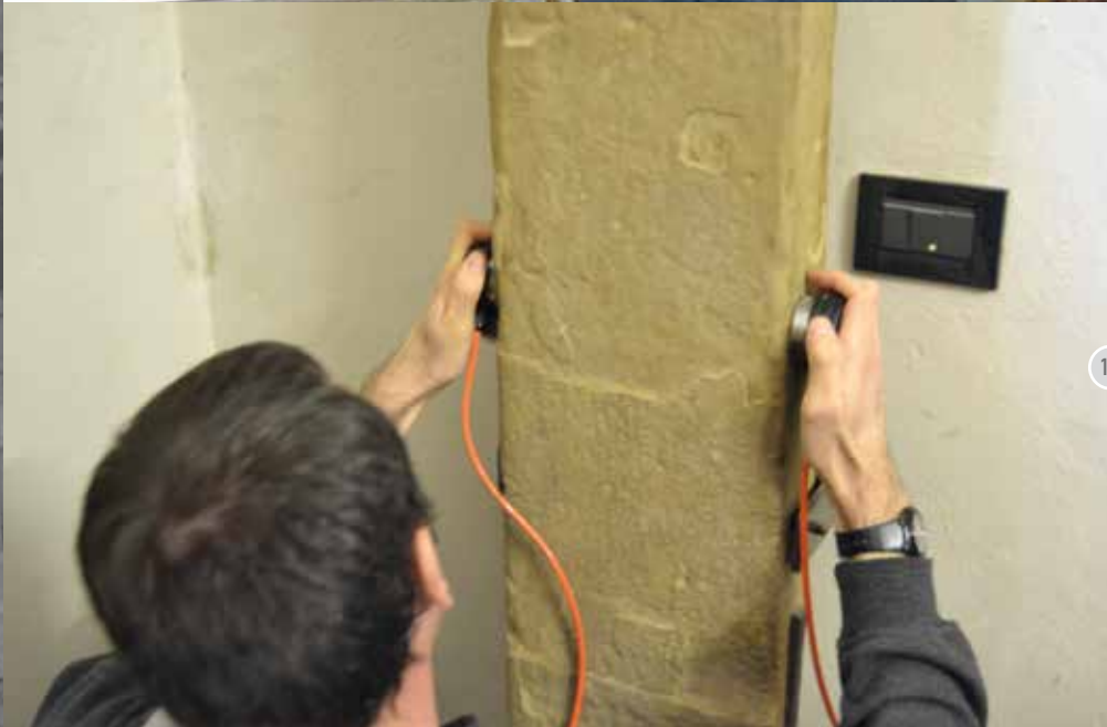
Fig 10. Relativity to the stone Cross, the application of direct ultrasonic survey reveal internal inhomogeneity of sandstone: a minimal degradation that testifies excellent storage condition considering his date of accomplishment
