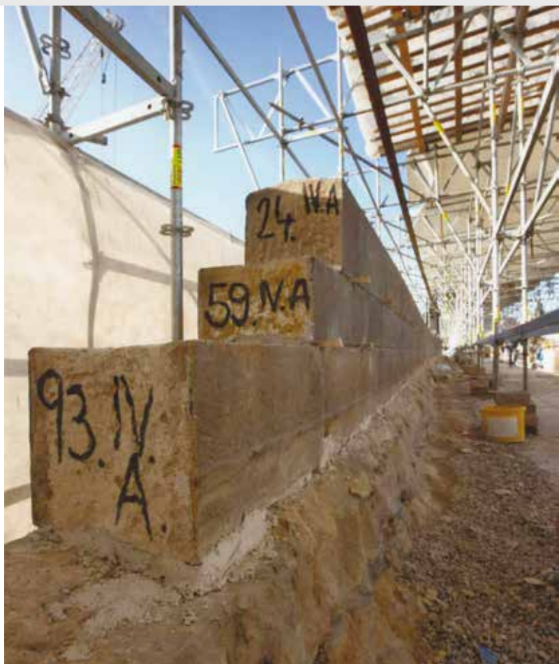
The Charles Bridge is made of blocks from different types of sandstones which make the framework and were carefully analysed. Damaged sandstone blocks were changed in the whole bridge cladding
